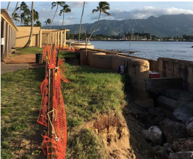
Temporary orange fencing was all that stood between the beachgoers and a collapsed bank in 2018. Photo: NSCC
