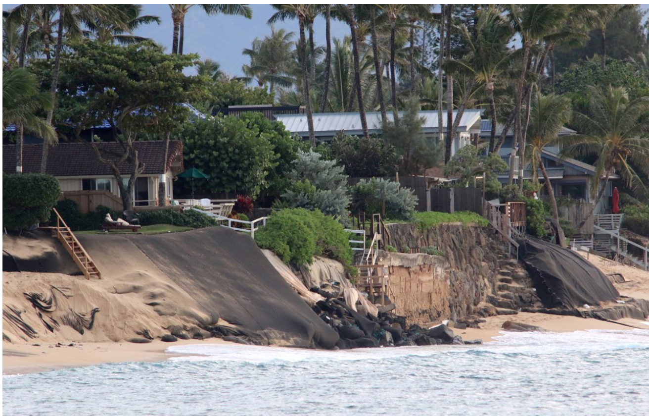
Erosion Rocky Point Area. Cover Story and Photos: banzaibetty.com
