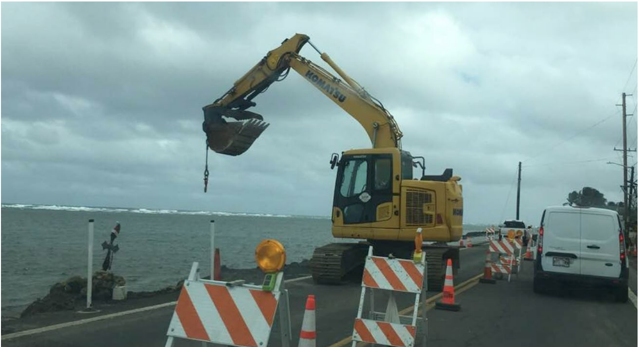
Department of Transportation repairing the damaged edges of the road in Hau’ula. Photo/Story: Choon James
