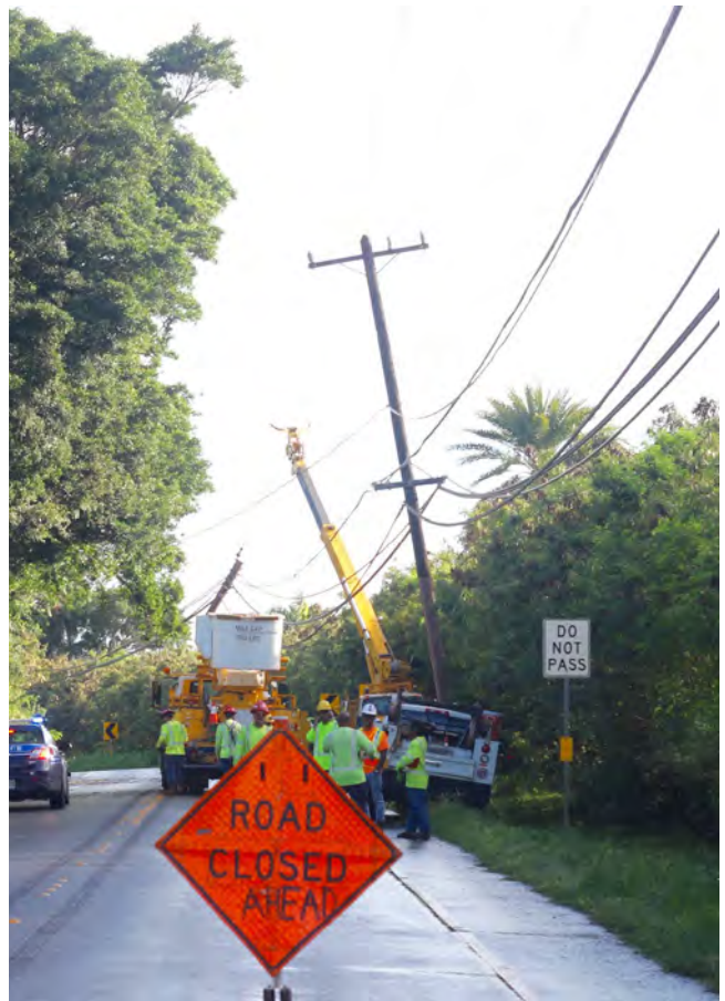
Utility pole down on Kam Hwy Photo: banzaibetty.com
