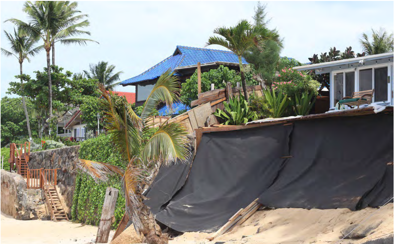
North Shore beachfront erosion Photo: banzaibetty.com
